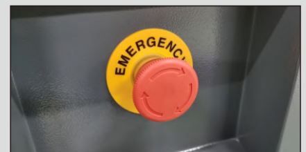
OUTSIDE EMERGENCY STOP
